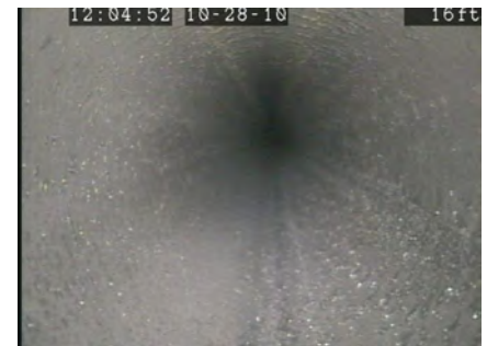
Same branch line with no corrosion, water filled with no air-water interface
