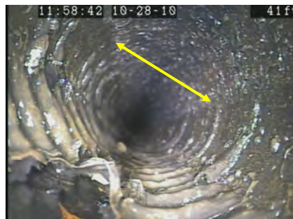
Branch line with significant corrosion deposits, clear air-water interface
