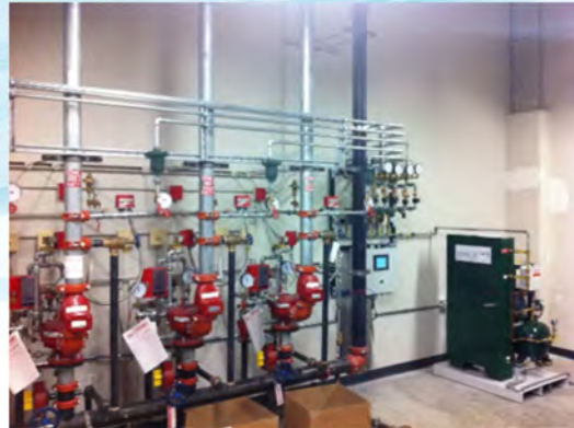
Nitrogen Generator installed in Riser Room
