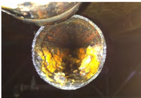
Corrosion at Air/Water Interface
