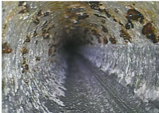
Galvanized Pipe Corrosion under Trapped Water
