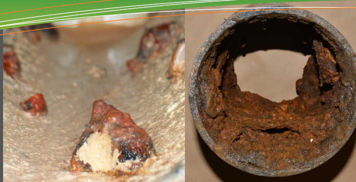
Left: tubercule on galvanized pipe from dry system Right: corrosion deposits on black steel in wet system
