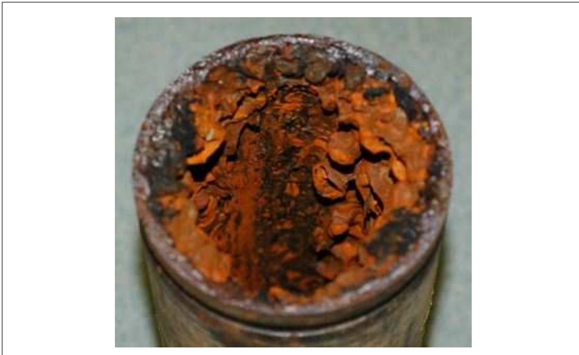
Fig. 15. Corroded steel pipe with many tubercles inside
