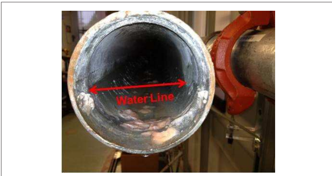
Fig. 4b. Galvanized steel pipe half-filled with compressed nitrogen after nearly six weeks' exposure
