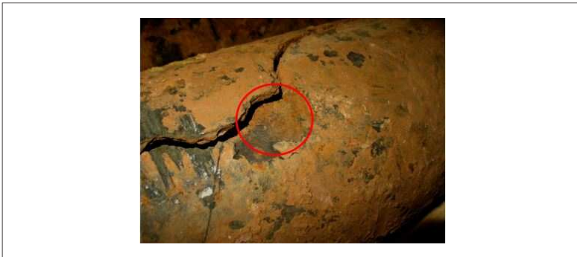
Fig. 7. Ruptured underground water main (identified as gray cast iron, 8 in. [20.3 cm] diameter) with cement lining on its inside diameter
