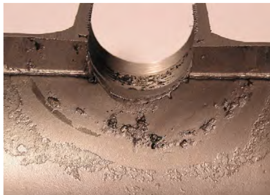
Anodic hot spot due to weld-o-let installation
