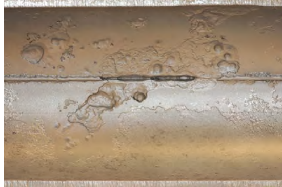
Knife cut corrosion on submerged weld seam (galvanized steel pipe)
