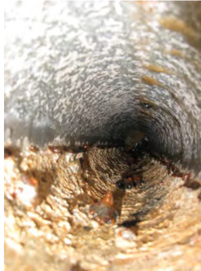
Evidence of trapped water in piping
