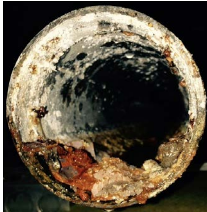
Figure 2: Galvanized Main Subjected to Oxygen Corrosion in Dry Pipe System
