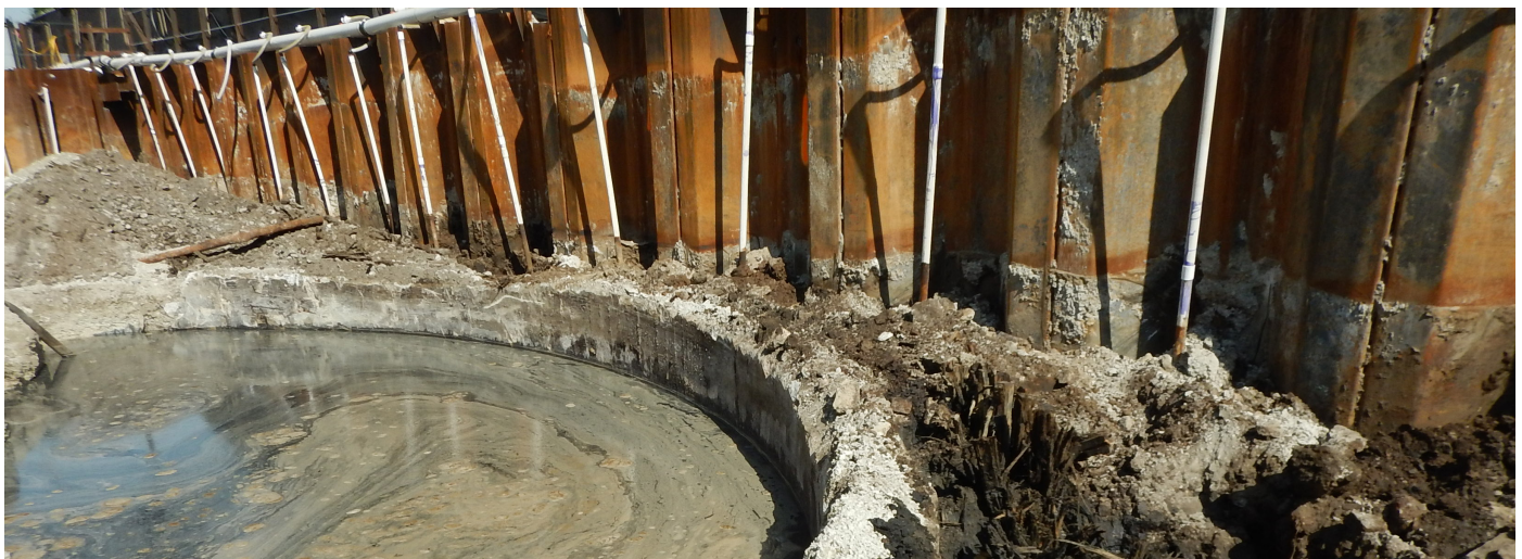
Sheeting design required a multiphase dewatering system, which generated significant quantities of impacted water to be pre-treated.
