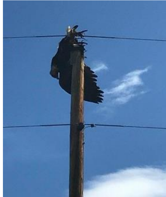
Single phase with ground wire at top of pole
