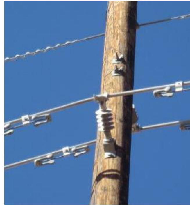
Short post-mounted insulators with ground wire bonding
