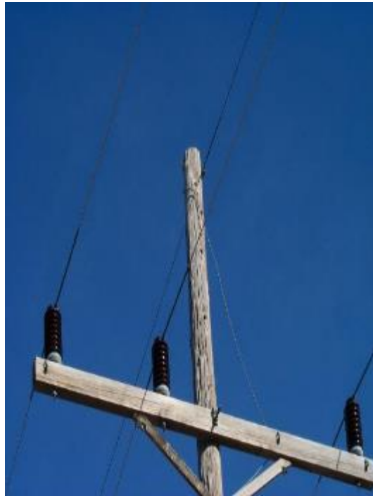
69-kV, 3-phase on crossarm with neutral along side of pole
