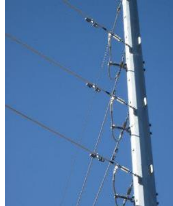
Short standoff insulators on jumper wires of angle steel pole
