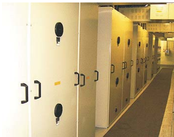
High voltage distribution equipment with infra-red portals.
