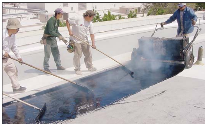
FiberTite fleece back being applied with hot asphalt over a BUR system
