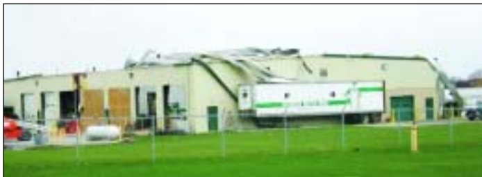
Wooster Motor Ways: Rated by the National Weather Service as an F-2 tornado with winds between 75 and 110 mph, the twister wreaked havoc on many industrial and manufacturing facilities in Wooster.
