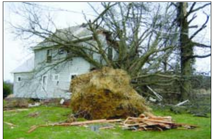
This residential property, located on the west side of Wooster, fell directly in the tornado's path of destruction.
