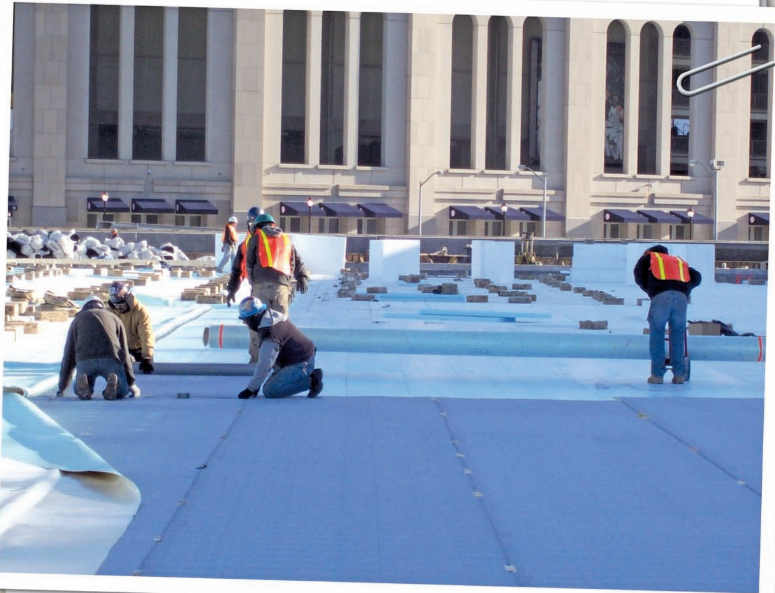
A 45-mil thermoplastic single-ply roofing system was installed over layers of polystyrene insulation and functions as the primary barrier to puncture from garden roots, hardscape, and park traffic.
