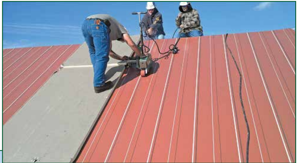
Photo 12 – Working with a preprinted metal profile illusion on a fluoropolymer roofing membrane.
