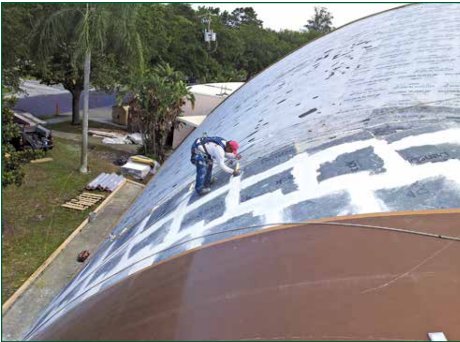
Photo 14 – Substrate preparation and grouting of the underlayment on Beth El Temple, shown in Photo 1.
