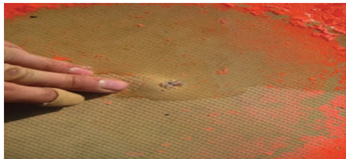
Exposed TPO Reinforcement Due to Polymer Degradation
