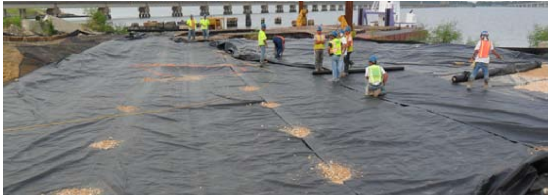
Engineered Textile Products built a decontamination station in Biloxi, Mississippi, using Seaman Corporation's 30-mil reinforced XR-5® geomembrane.
