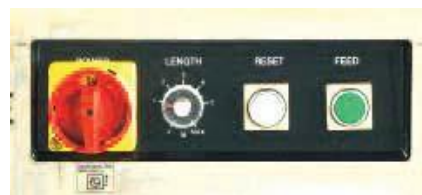
OPERATOR FRIENDLY CONTROL PANEL
