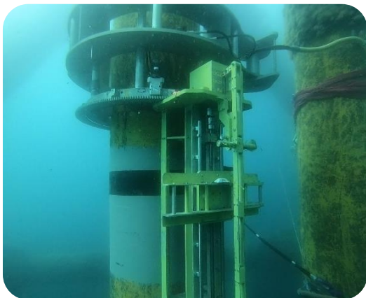
Existing wrapping machine
