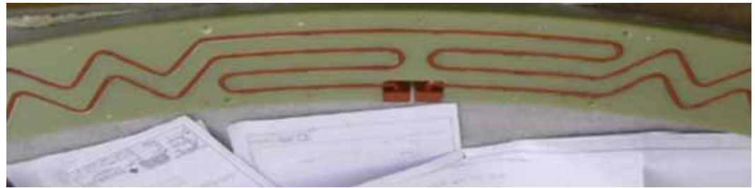
Coil mounted underneath a conveyor for heating metal cans.
