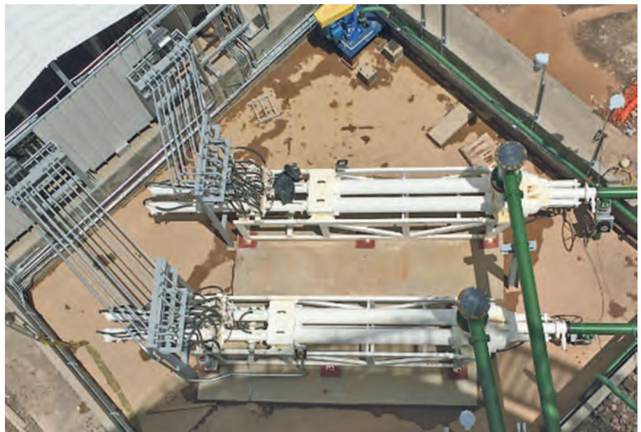
Schwing Bioset KSP440 piston pumps at Rumichaca tailings site, Peru
