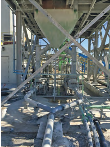
New and improved paste plant at San Jose mine with Schwing Bioset KSP80 pumps
