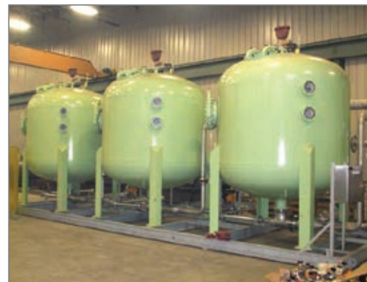
Industrial Process Water Treatment
