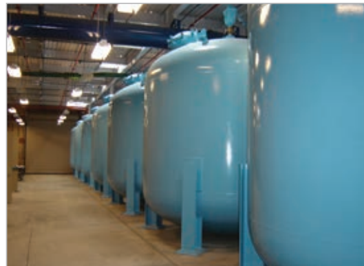
Municipal Water Treatment
