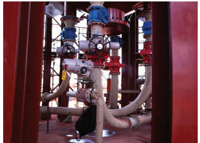
Underflow Control System
