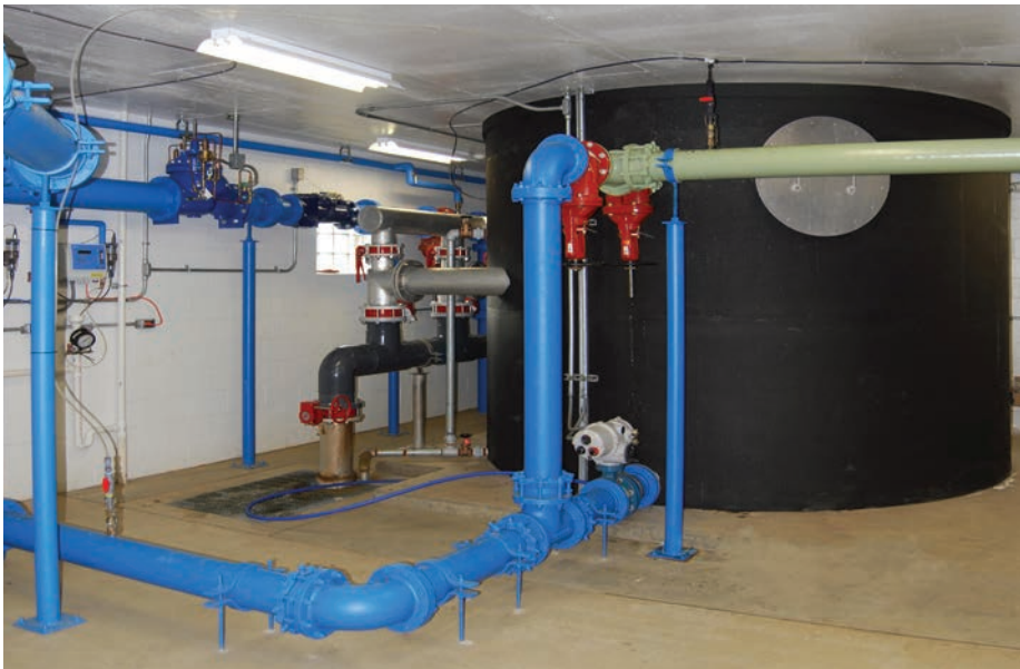
The visible section of the AERALATER is covered with insulation to minimize condensation.
