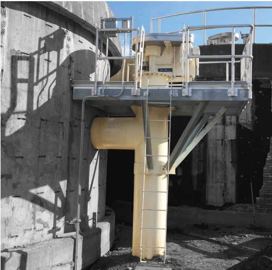
External ExtremeDuty sludge mixers
