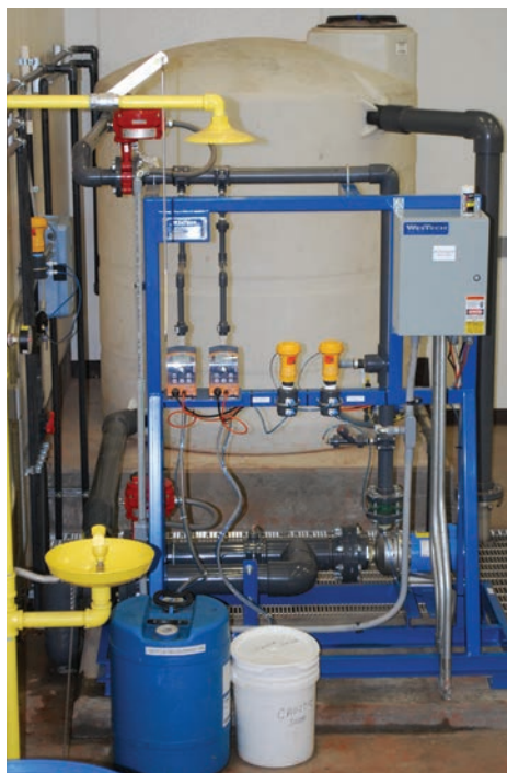
An optional neutralization system was included with this equipment to allow for discharge of chemical solutions used during membrane cleaning.
