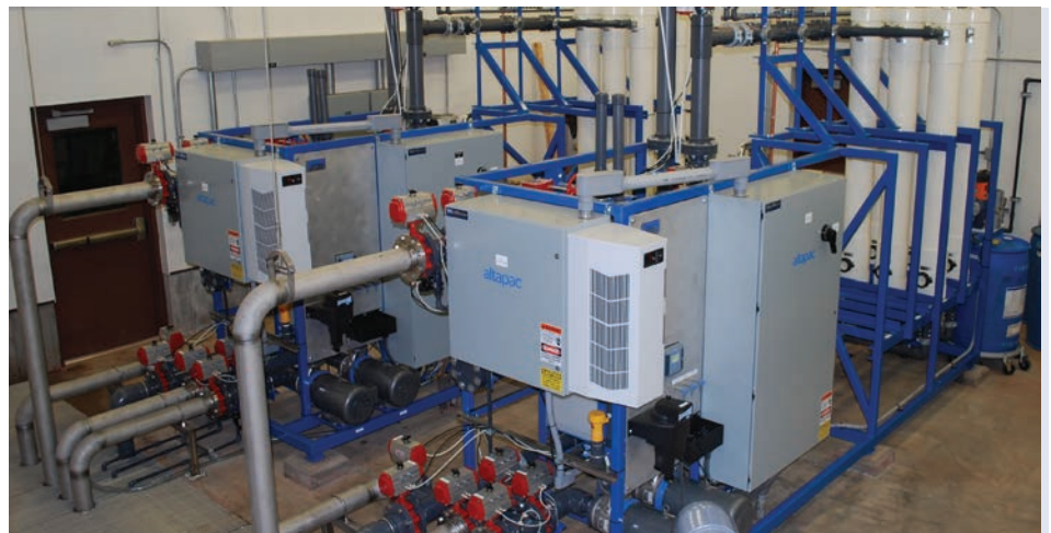
The compact and efficient design of the AltaPac limited the costs of installation and construction of the new treatment building.
