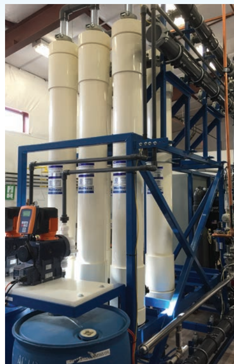
Only half the ultrafiltration racks are populated due to current demand. The capacity of the system can be doubled quickly and inexpensively by installing additional modules. All system components are sized for the increased capacity to limit costs associated with expanding the system.
