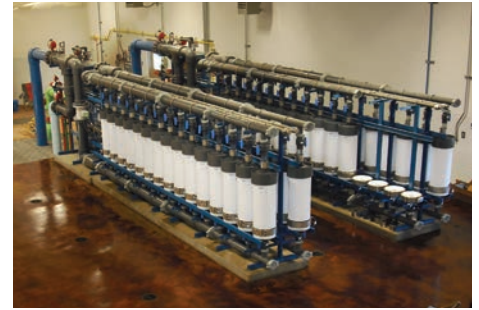
Ultrafiltration Membrane Filter Trains
