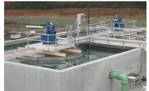
Solids CONTACT CLARIFIER™
