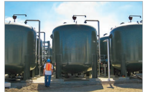
Vertical Pressure Filters at Westminster Well Site
