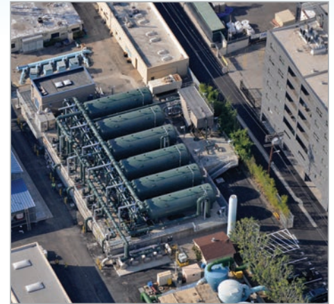
Horizontal Pressure Filters at Bundy Well Site
