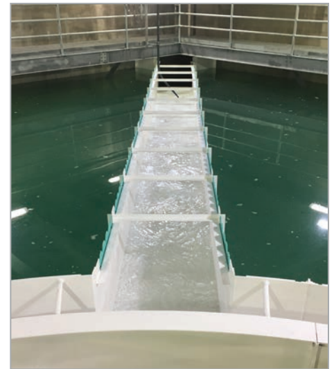
Solids CONTACT CLARIFIER in Production
