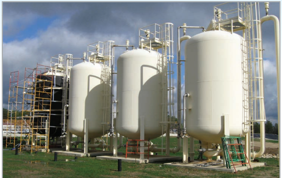
Granular Activated Carbon Pressure Filters
