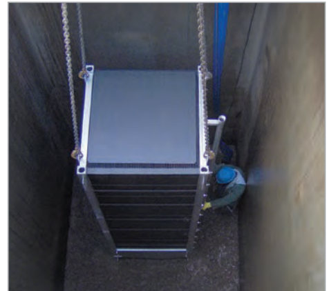
ClearLogic® MBR Installation
