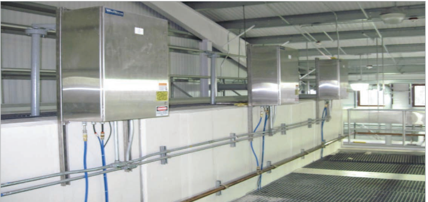
With the help of the SuperSand filters, Peach Lake Environmental Center exceeded requirements for discharge of wastewater into the lake, preventing its further contamination.
