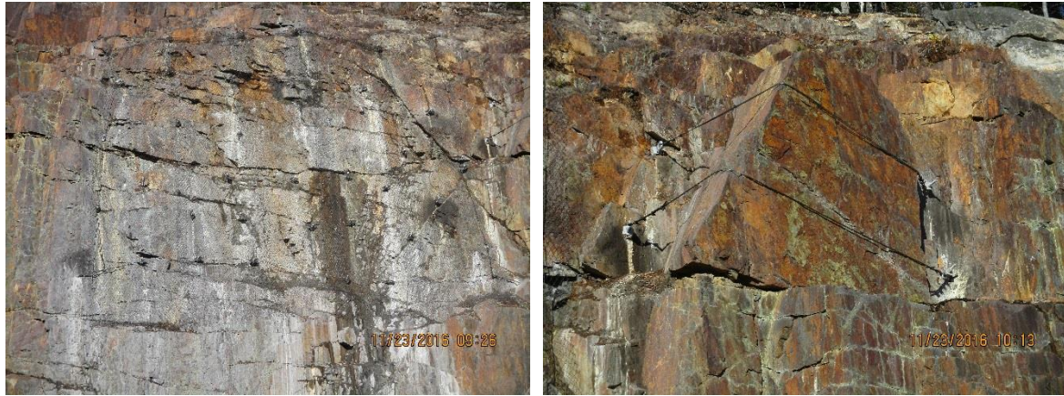
Figure 12 – Wire Mesh Netting and Wire Rope Cable Lashing in Areas 5 and 5A
