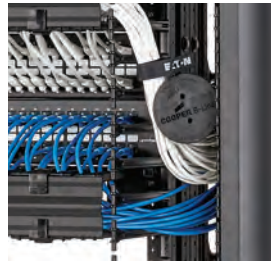
Telescopic Cable Spool To Manage Bulk Cabling
