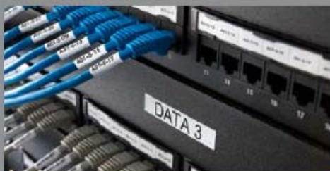
Wire & Cable Identification
