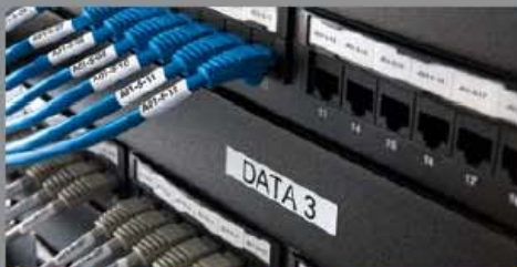
Wire & Cable Identification
