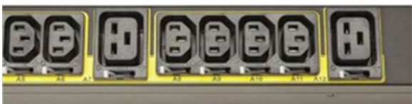
Figure 1. Rack PDUs with IEC outlet grips can reduce the risk of plugs getting bumped loose and leading to server shutdown.
