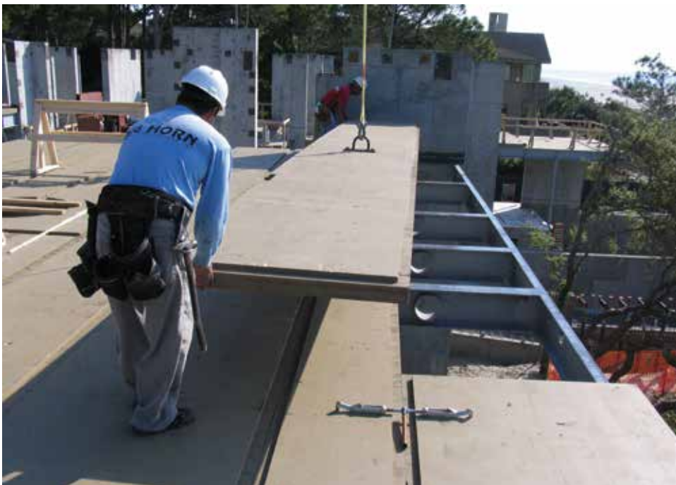
Figure 7 Lifting and handling of CLT elements in an hybrid structure, in the United States (courtesy of Binderholz)
