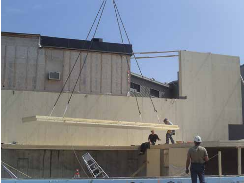
Figure 6 Lifting and handling of CLT elements, in Canada (courtesy of KLH ELEMENT, photo: © Marc Cramer)
