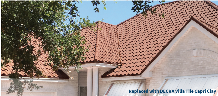
Clay tiles struck by hail.
