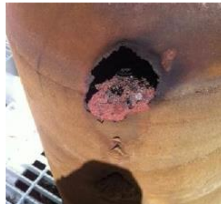
Figure 2 Partially melted foam pig.
