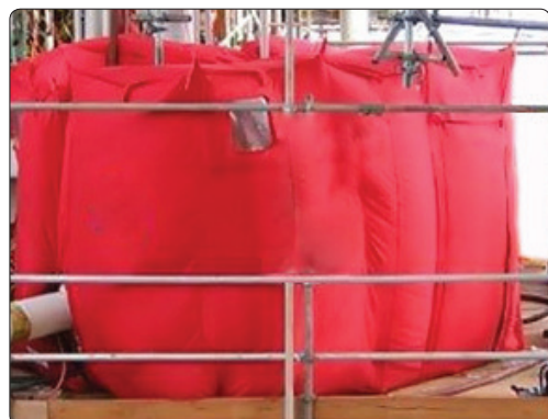
Typical welding habitat
