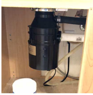
Sink / Faucet (4/5) 05/31/2019 8:11 AM
