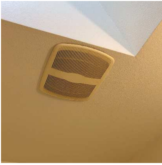
Exhaust Fan (2/3) 05/31/2019 8:32 AM
