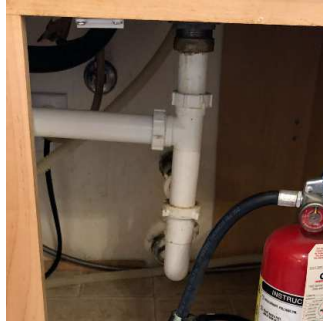
Sink / Faucet (5/5) 05/31/2019 8:12 AM
