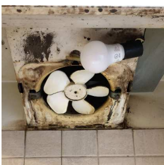
Exhaust Vent 05/31/2019 8:11 AM
