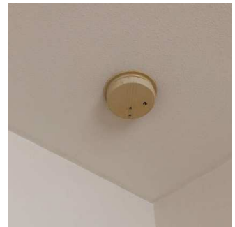
Smoke Detector (2/3) 05/31/2019 8:28 AM
