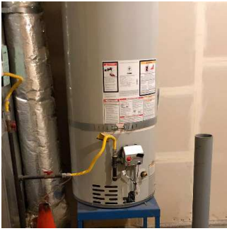
Water Heater (1/2) 05/31/2019 8:17 AM
