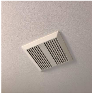
Exhaust Fan (3/3) 05/31/2019 8:38 AM
