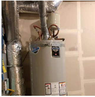
Water Heater (2/2) 05/31/2019 8:17 AM
