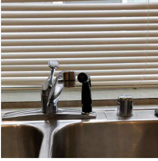
Sink / Faucet (3/5) 05/31/2019 8:11 AM
