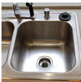
Sink / Faucet (1/5) 05/31/2019 8:11 AM
