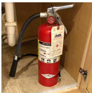
Fire Extinguisher 05/31/2019 8:12 AM
