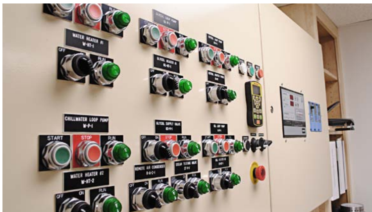
Wind Tunnel Control Panel Instrumentation
