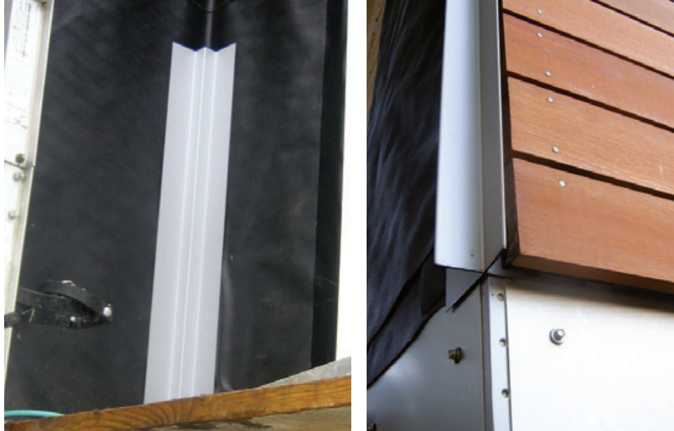
Figure 3. A custom sheet-metal shop fabricated battens and metal trim elements for the project, including inside corner trim (far left) and X-profile outside corners (left). The horizontal aluminum “belly band” was fastened to the sheathing with gasketed screws, which were driven into slightly oversized holes to allow for thermal expansion of the metal.
