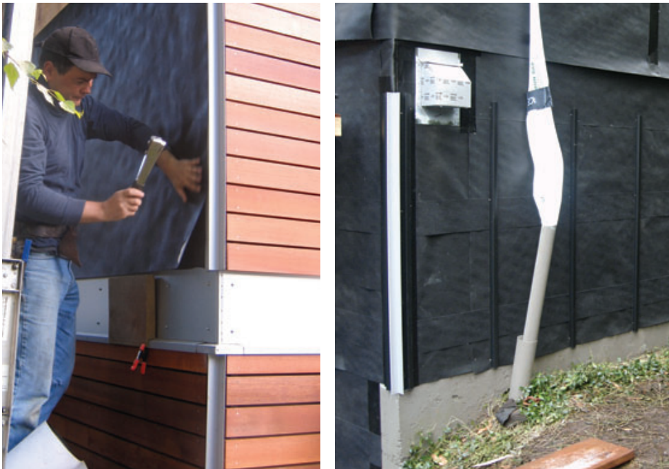
Figure 2. With narrow siding, such as these 4-inch cedar boards, two full layers of underlayment were required for UV protection (far left). Where wider panel siding was used, a full single layer was applied, followed by 6-inch strips beneath panel joints (left). The vertical “streamer” is a temporary sheet-plastic downspout.
