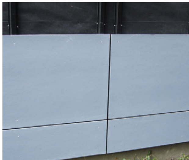
Figure 4. Fiber-cement wall panels were fastened with ring-shank stainless nails. Two battens were used at vertical joints, one on each side of the gap.
