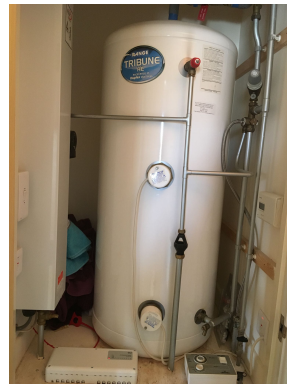
Domestic Hot water
