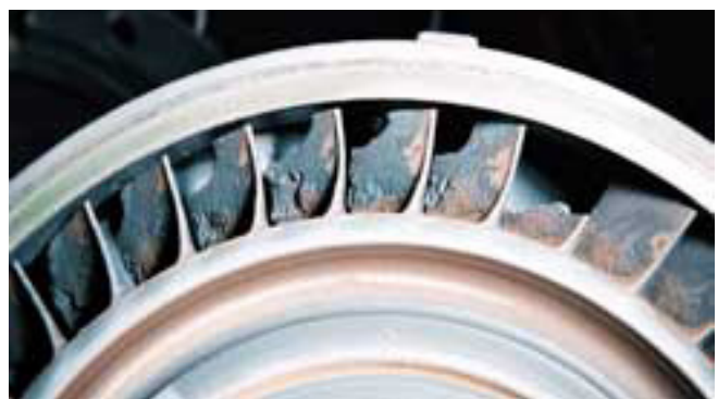
Figure 4: Severe sulfidation corrosion on turbine blades leads to lost efficiency and blade failure.
