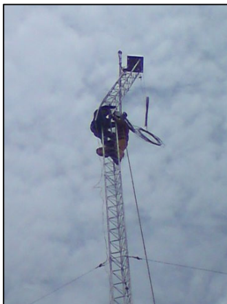
SAC Installation Site in Malaysia
